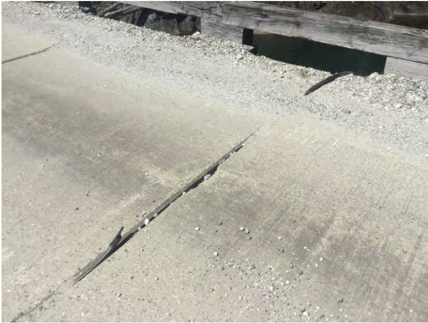
Failed Compression Seal
