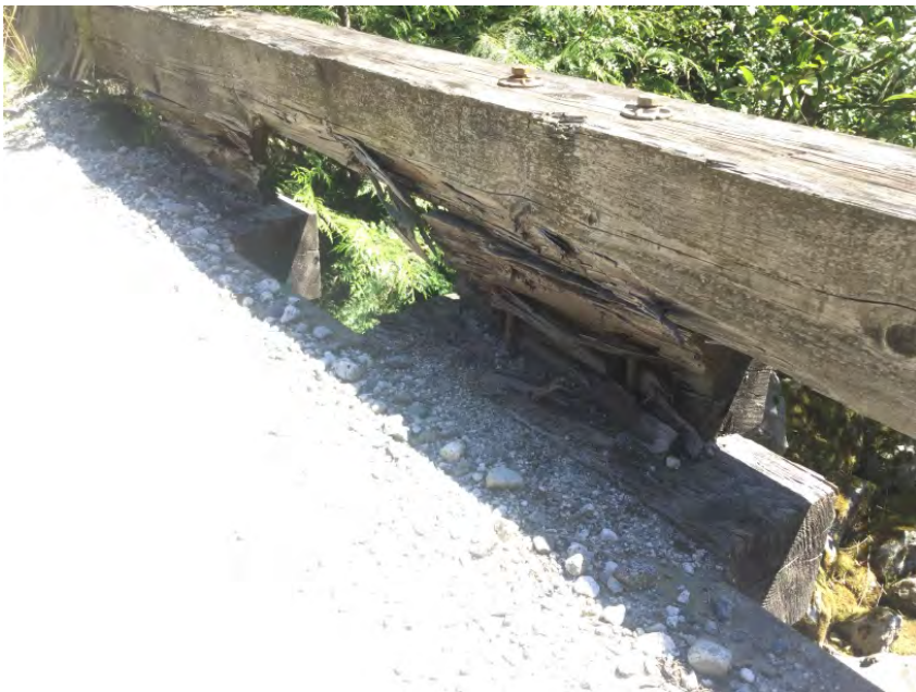
Left Abutment Downstream Corner Rotten Risers
