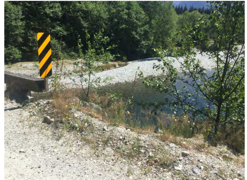
Right Approach Downstream Corner Missing Fender
