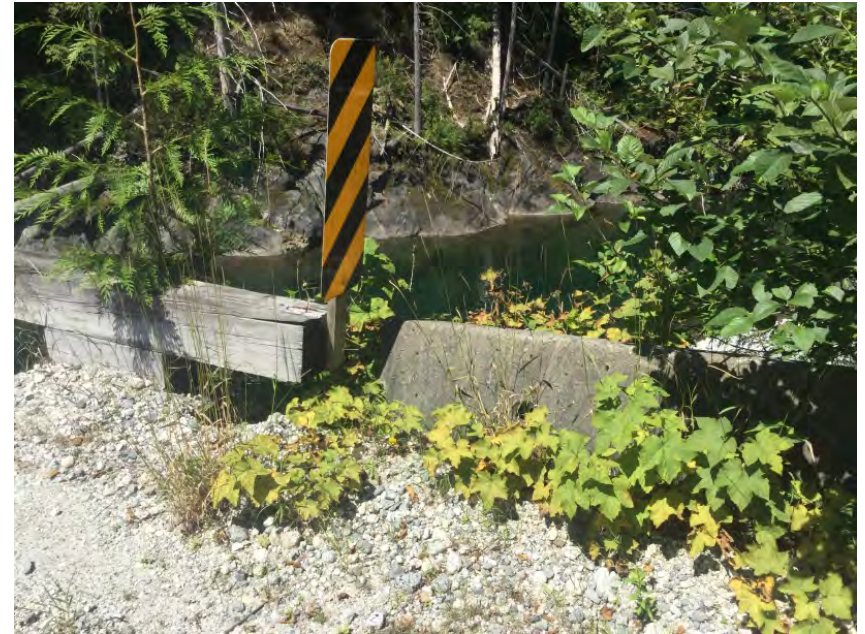
Left Approach Upstream Corner Partially Overturned Fender
