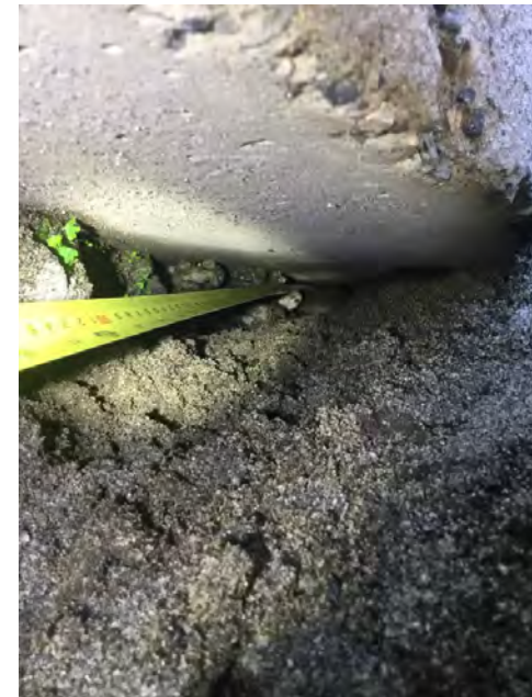
Right Abutment Downstream Footing Scour
