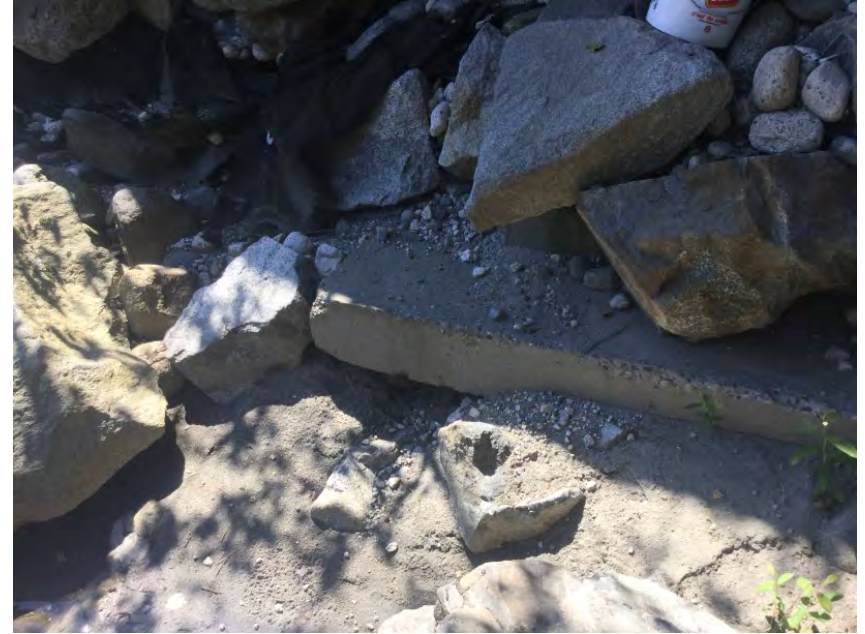
Right Abutment Downstream Footing Scour
