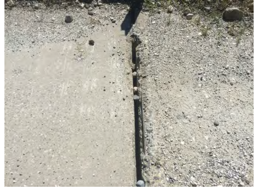
Right Abutment Damaged Ballast Wall in Wheel Track
